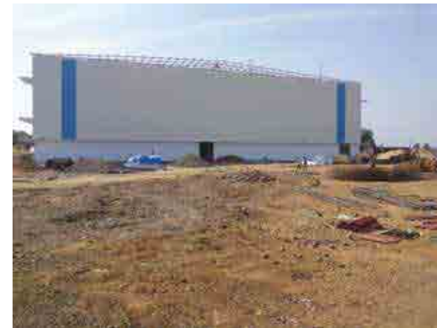
USED IN WAREHOUSE
